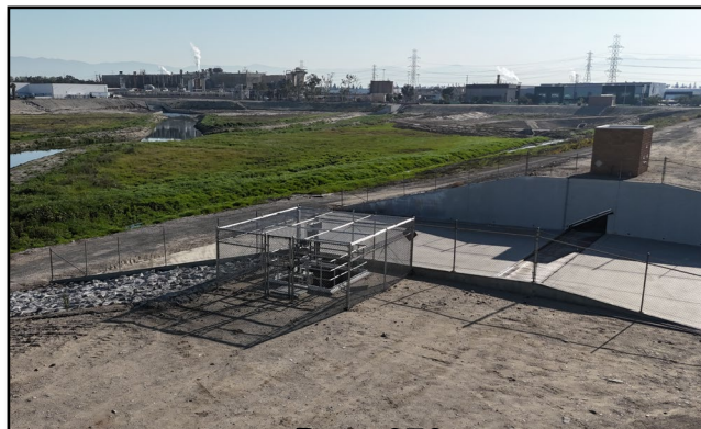
Page 376 Outlet Control Gate/Rubber Dam System
